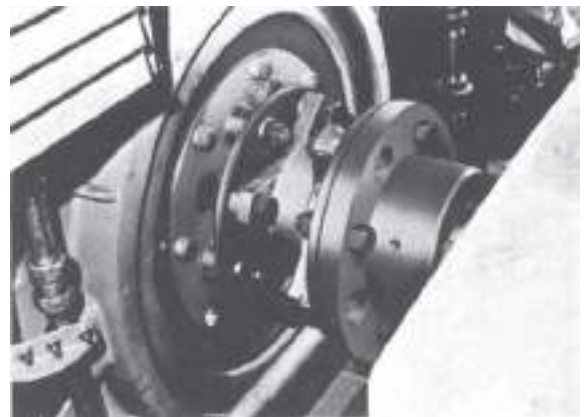
CMR coupling between engine and reciprocating compressor.
